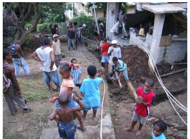
Figure 2 Action-to-Knowledge (A-K): Community residents commencing drainage construction in a vulnerable community in which houses had previously been destroyed by landslides.
